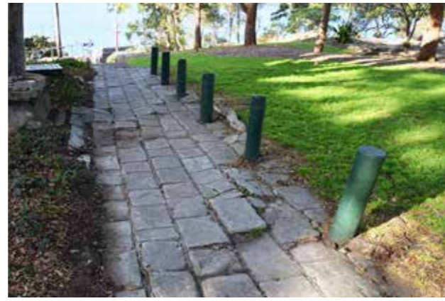
Existing broken flagstone path to ferry - remove bollards
