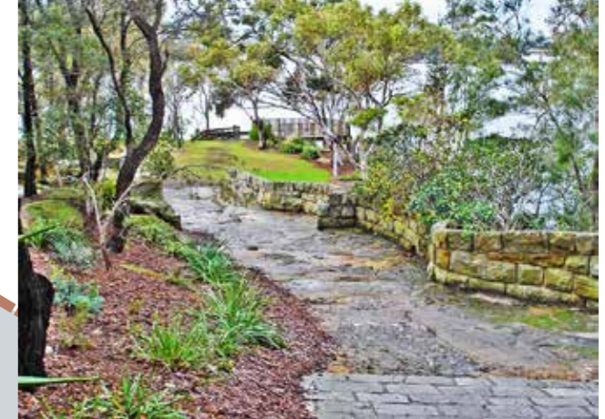
Shallow rock scabbling required to establish a smooth alignment for the new stone path. Remove the first few courses to help re-align the new paving junction
