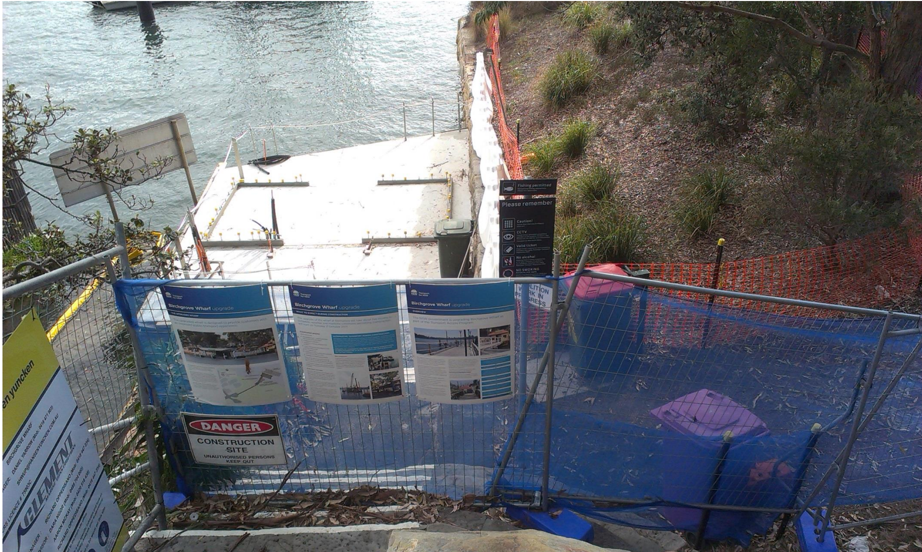
New wharf platform with waiting shed footings viewed from stairway. Option for access ramp trench through retaining wall and garden to the right
